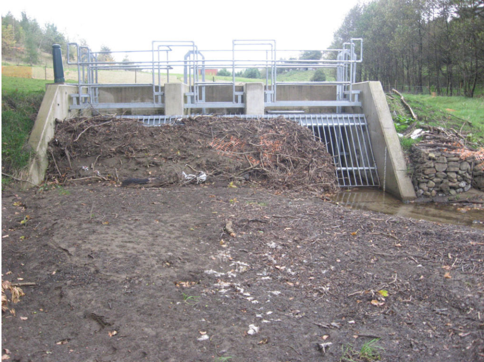
Blocked grid following heavy rain
